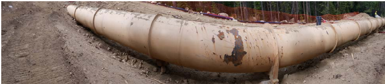
Buried pipeline had been excavated to expose corrosion and allow for repair work
